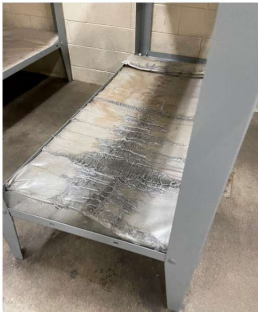
Figure 4. Severely Worn Sleeping Mat at Chula Vista Border Patrol Station, Observed May 18, 2023
