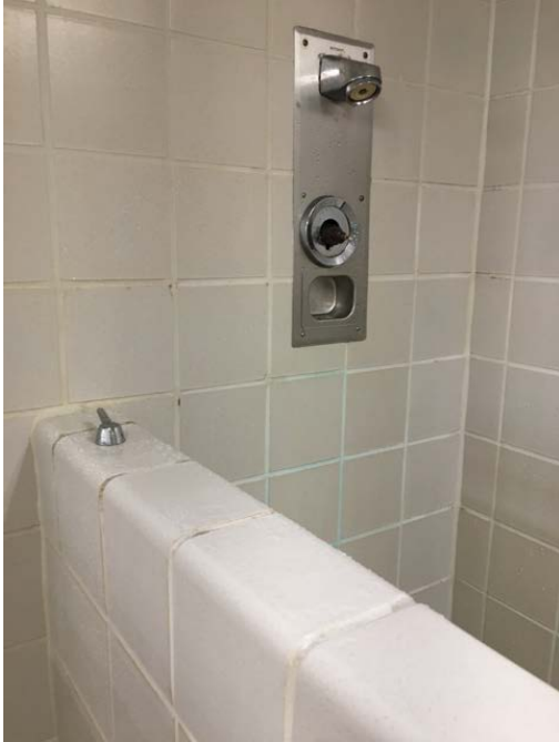
21 Broken detainee shower handle
