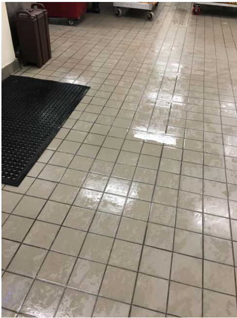
12 Water puddles on the kitchen floor
