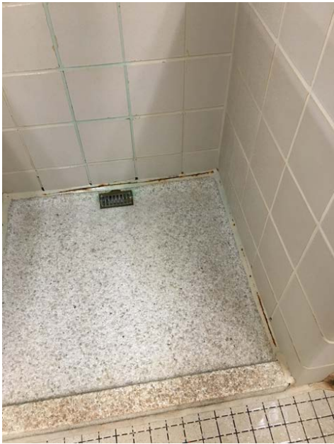
20 Grime/mold in detainee shower area
