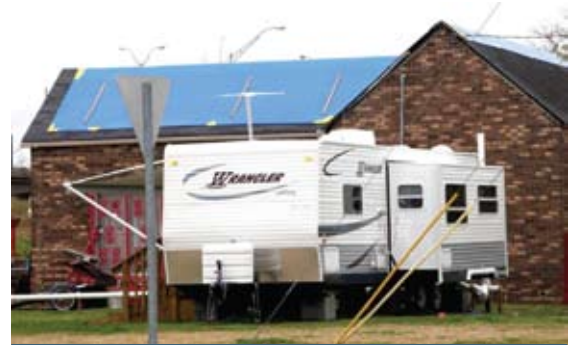
FEMA trailer and house with "Operation Blue Roof" Tarp
