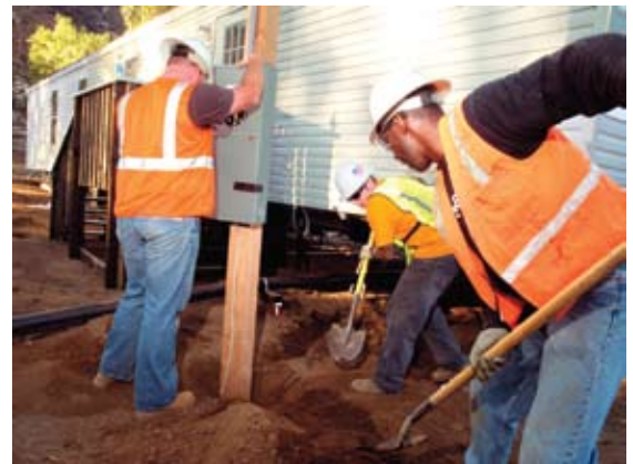
Delzura, CA., December 5, 2007—The electricians are hooking up electricity to serve a family that will temporarily live in the FEMA-provided mobile home while they begin to rebuild. The family lost their home during the wildfires in October.
